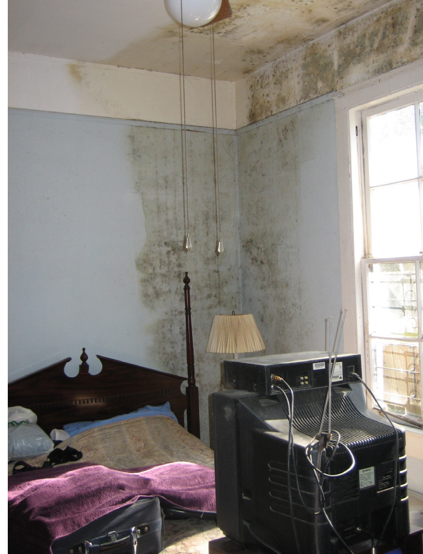
Pictured: A house in the predominantly Black city of New Orleans after Hurricane Katrina caused mass flooding, over 1,000 fatalities, and $108 billion (unadjusted 2005 dollars) worth of damage in 2005. This house was evacuated and left for two weeks, during which time visible mold manifested due to serious leaks in the exterior. (Infrogmation, 2005). CC BY-SA 2.0. [38]
